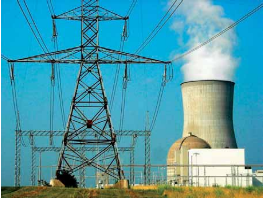
FIG. V-4. Power lines coming into the Callaway NPP.
